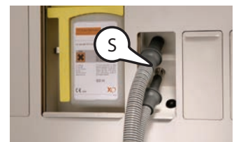
Suction hoses fitted at disinfection nipples.
